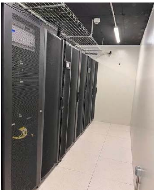
Figure 5: Interior view of the EOLAB Data Centre.
