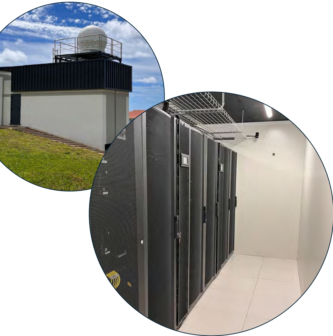
Figure 2 AIR Centre Data Centre in Terceira Island.
